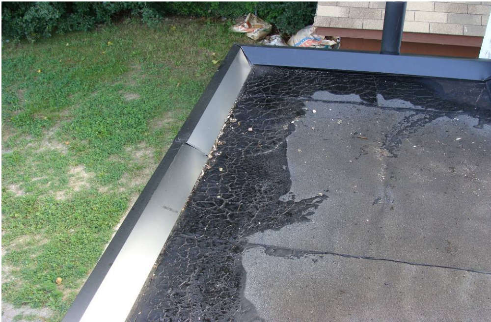
Photograph 8: View of the hot pour asphalt repairs at the low roof area.
