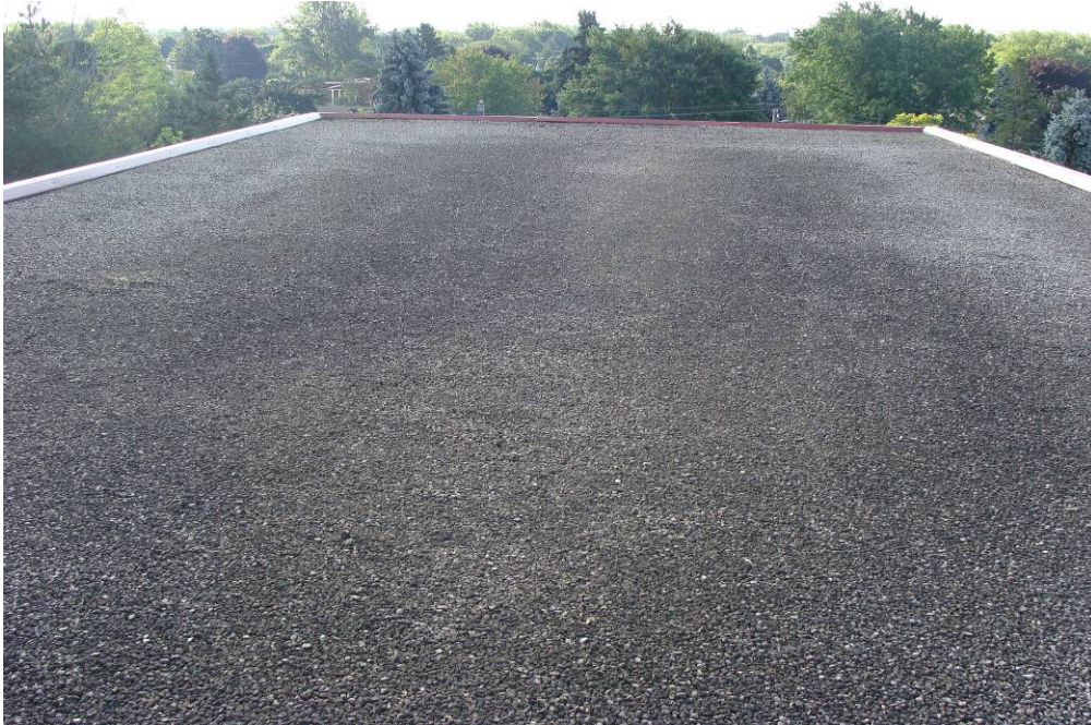
Photograph 1: View of the main roof area. The dark areas in the gravel surfacing indicate areas of ponding water.
