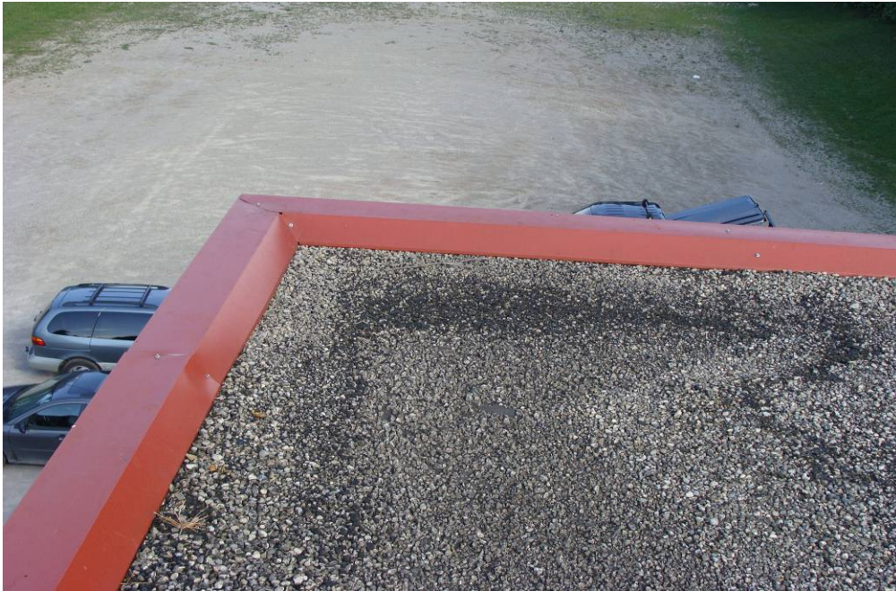
Photograph 3: Scouring at the corner of the roof area, exposing the membrane.
